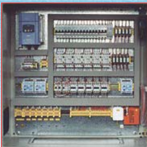
Control system of the set of six 3kW pumps.
