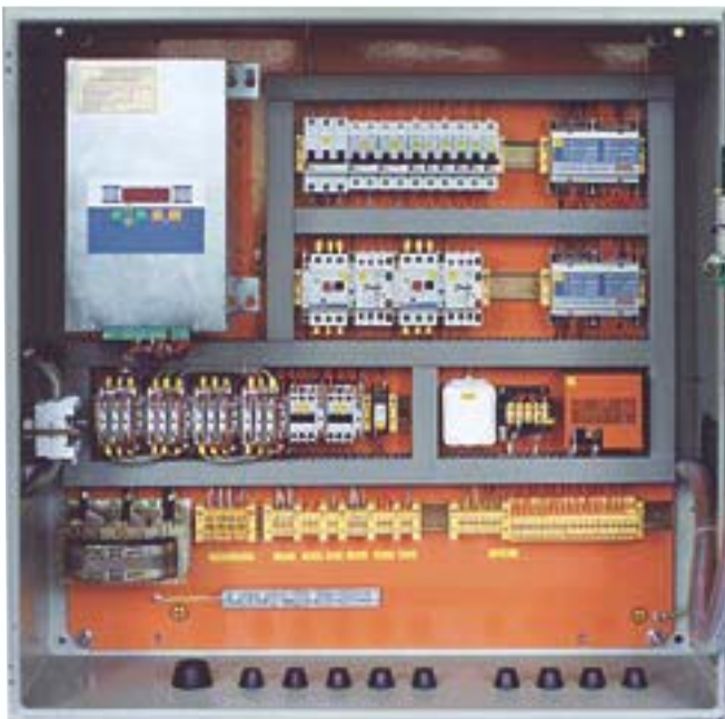
Interior of a switchbox controlling two 15 kW blowers.
