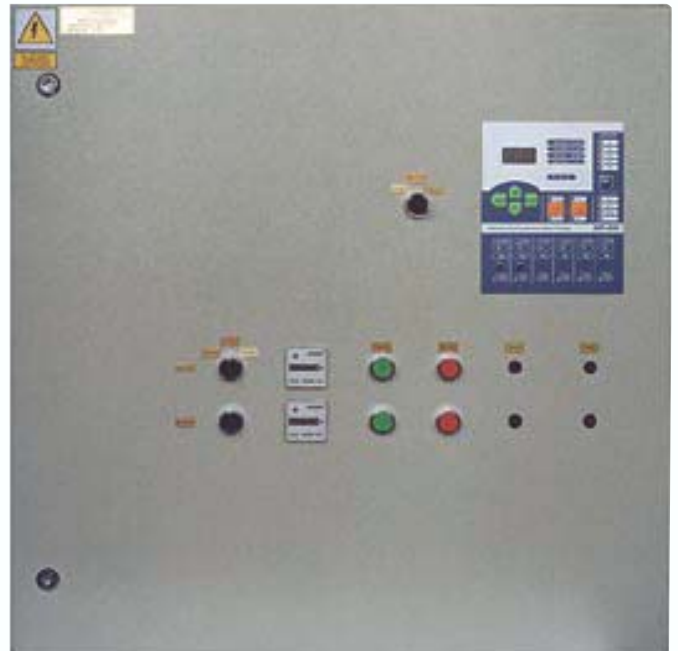
The front of a switchbox.
